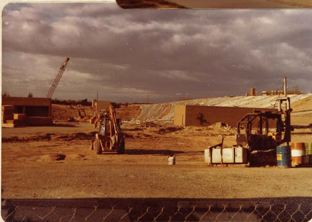
Still under construction is the California Bowl, the new stadium located adjacent to the CSUF campus. Completion is set for 1980
